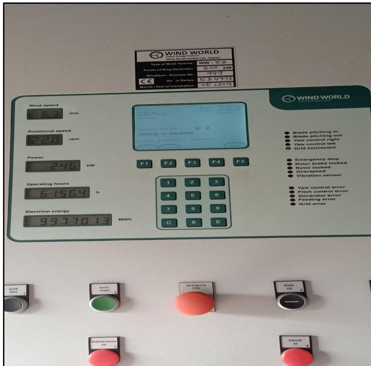
Figure-2: Control panel
